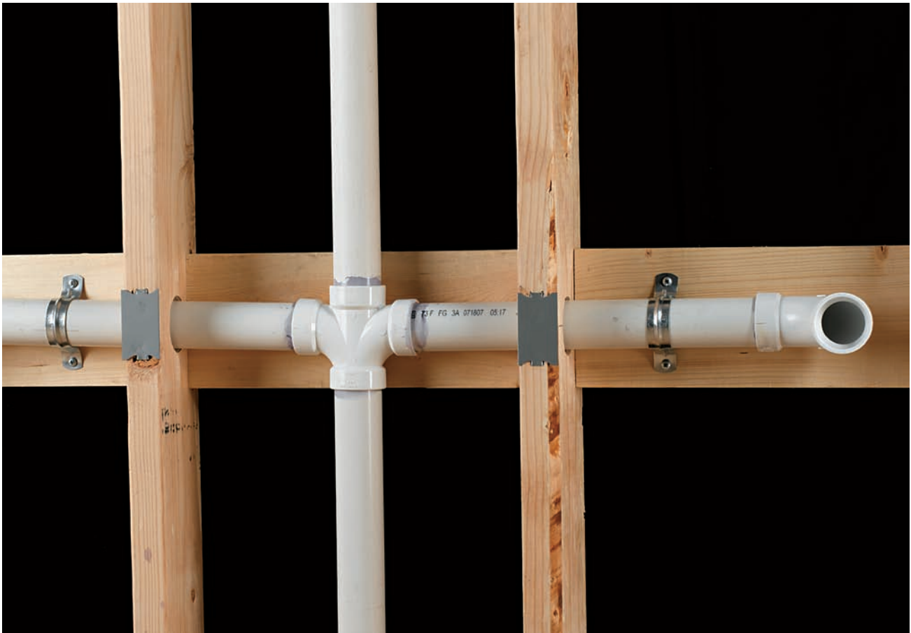
Common vent with vent connecting at fixture drain intersection.
