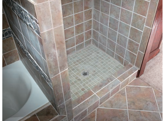
Showers & tubs. Provide at least 80" of finished ceiling height for all of the required floor area in showers and in tubs containing showers.
