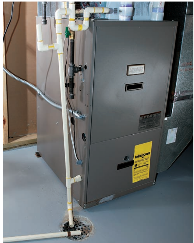
Condensate from air conditioner units should be directed to a drain through discharge pipes.
