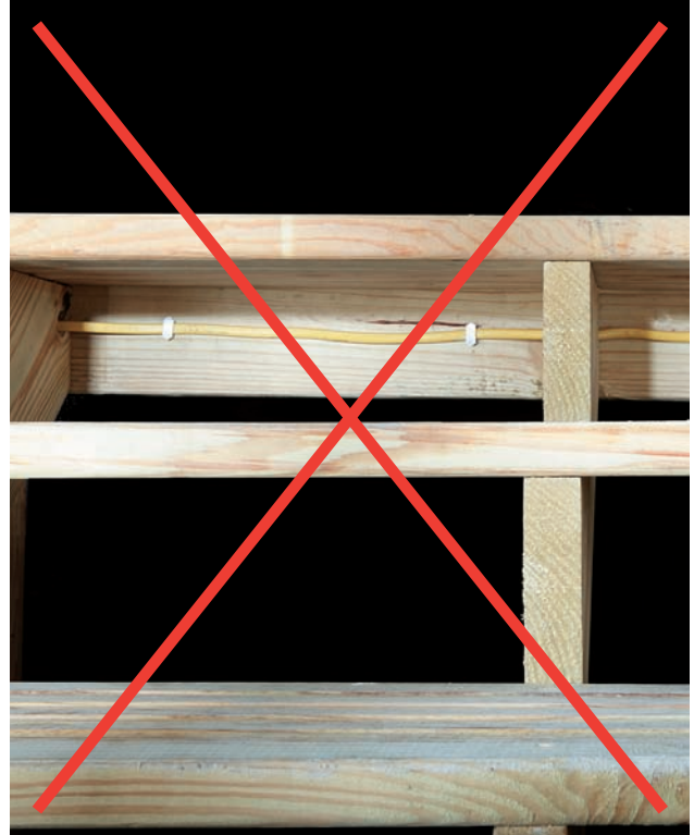
VIOLATION! Do not install NM cable outdoors. Outdoors includes buried conduit. You may install UF cable outdoors if it is protected from physical damage.
