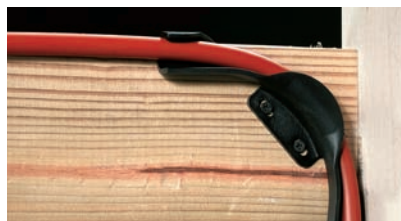
Support for PEX tubing is particularly important near manifolds and fittings.
