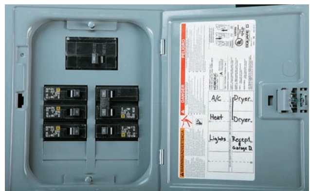
Label each circuit in all electrical panels so that the purpose of each circuit is clear.
