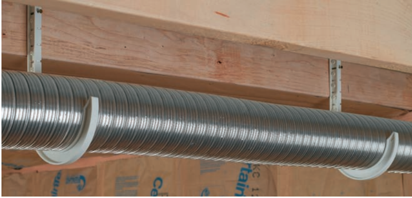
Intervals between supports (hangers) for flexible HVAC ductwork can be no more than 4 ft. apart.
