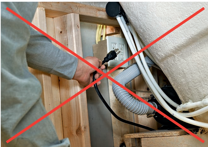
Receptacles for whirlpool tubs must be GFCI protected and must face the access opening. The receptacle shown here is a violation.
