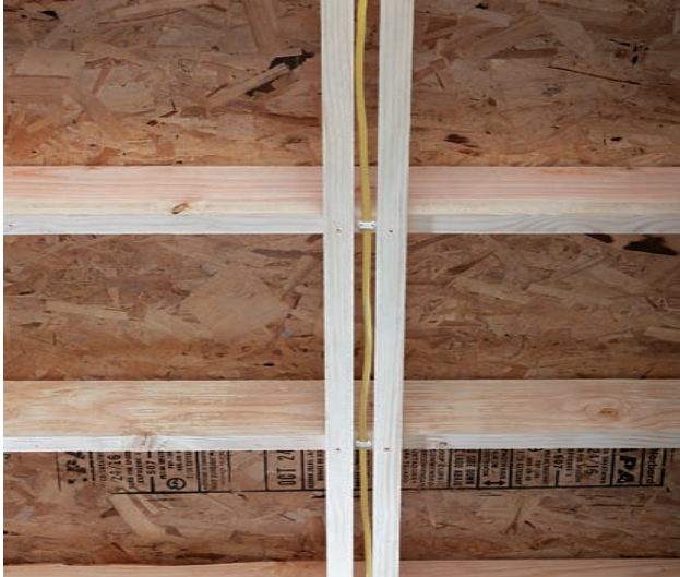
Use wood or other substantial guards to protect NM and UF cable installed perpendicular to rafters within the protection area.
