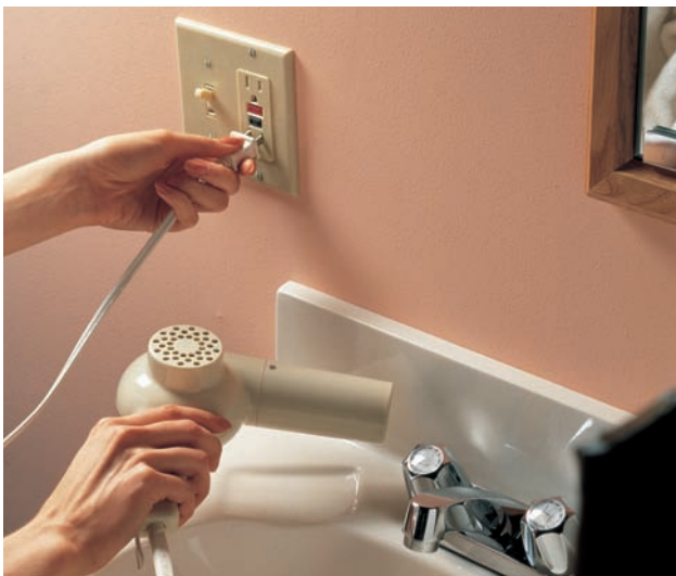
A GFCI protected receptacle must be installed within 36" of each bathroom sink basin.
