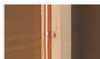
From the vertical support brackets hanging parallel to wall studs, first supports according to table 32.
