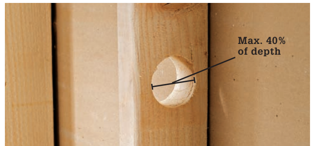
Drill a hole in a load-bearing stud not more than 40 percent of its actual depth.
