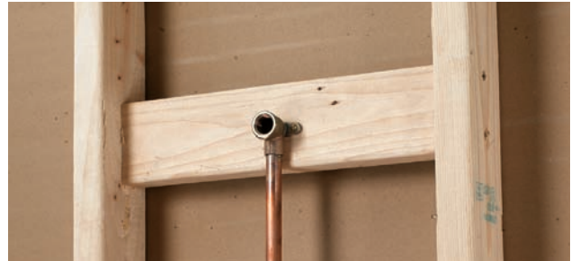
Attaching the shower riser pipe to framing helps avoid water leaks caused when adjusting the showerhead loosens the pipe fittings.
