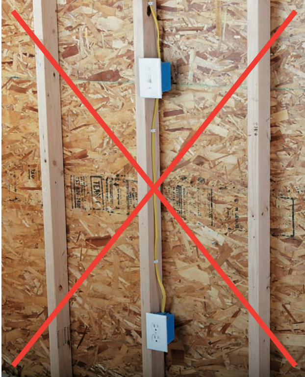
VIOLATION! Do not install NM and UF cable in exposed walls and ceilings. You may install NM and UF cable in exposed basement ceilings and attics under certain conditions.
