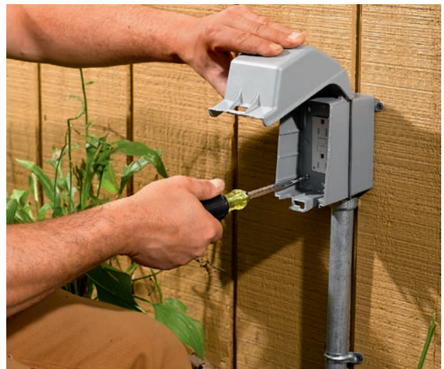
An exterior-rated receptacle should be installed on both the front and back exterior walls of your house.
