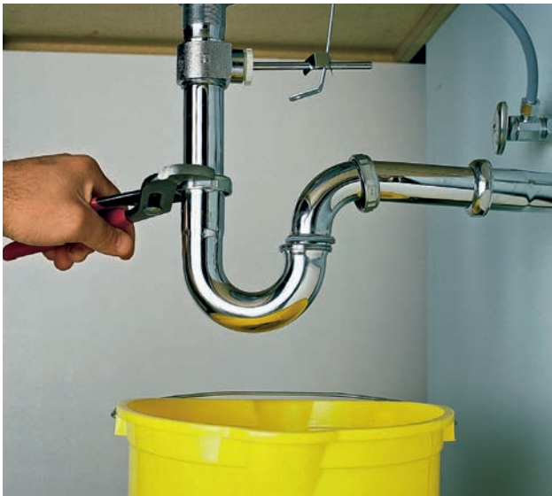
Chromed P-trap with slip joints on lavatory sink.
