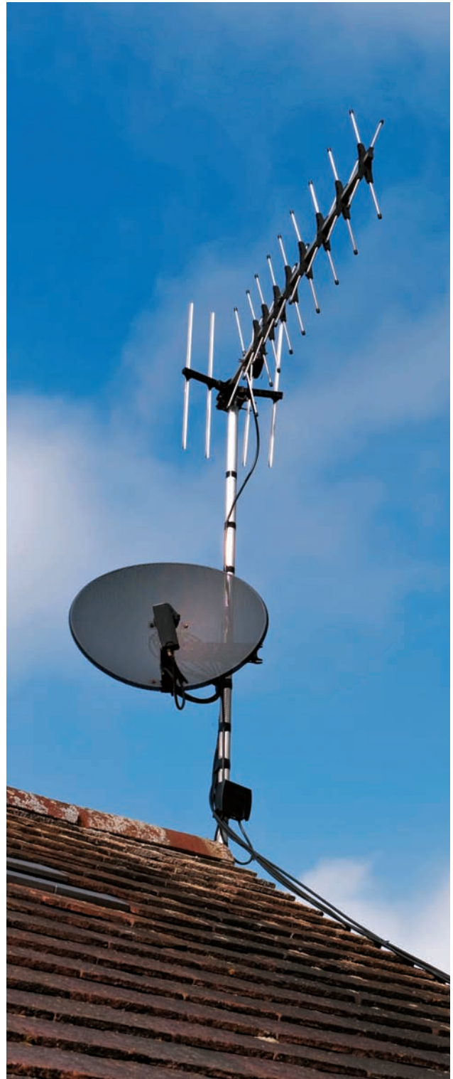
Television aerials and satellite dishes must be located well away from power lines. They should be properly grounded and protected against lightning strikes.
