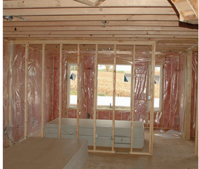
Even nonload-bearing walls must conform to construction codes.
