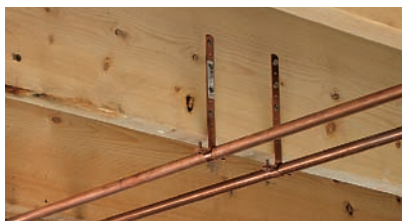
Support copper tubing with compatible hangers.
