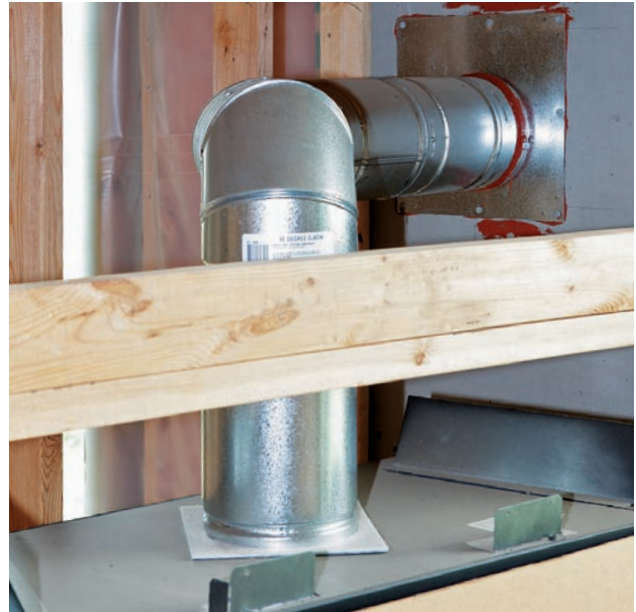
Direct-vent gas fireplaces may be vented through a sidewall. Chimneys for wood-burning fireplaces are vertical.
