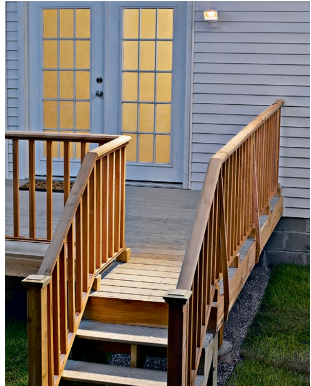
Install a light at the top landing of above-grade exterior stairs.
